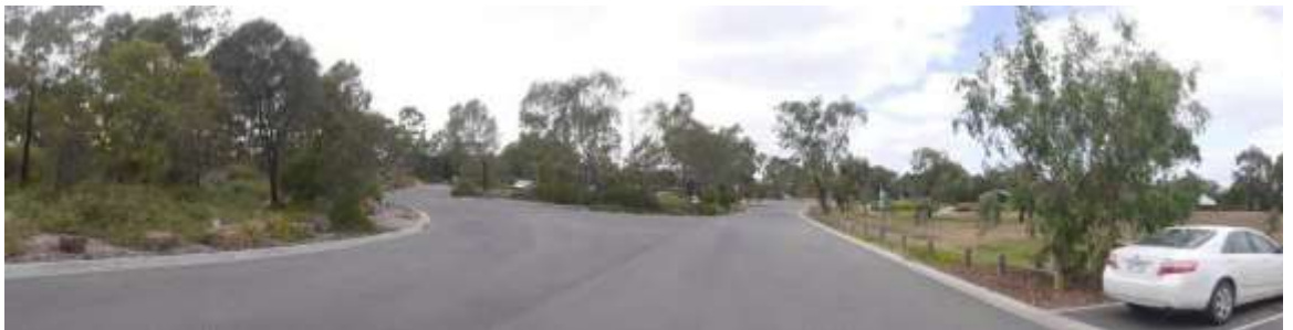
Photo 28: Main car park no directional marking
